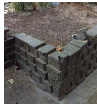
Unightly: Old and crumbling wall sections to be removed
