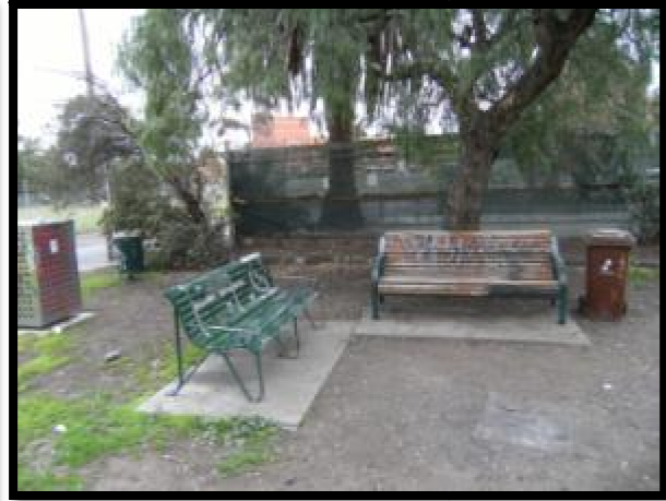
Figure 17: Graffiti damage to seating and bins
