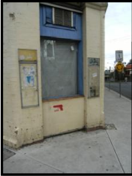
Figure 12: Badly maintained building, corner Buckley and Nicholson Sts
